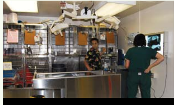
Animal Care & Control recently upgraded their veterinary facilities to meet state codes. The room contains a new sterile surgical suite and better equipment to help our veterinary staff do their best to help our shelter animals.
